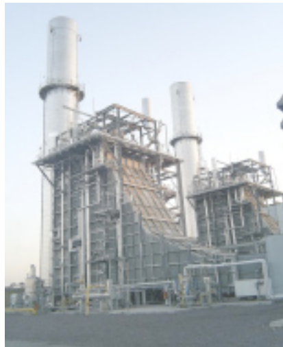
3. Dual-pressure HRSGs produce steam at 1465 psig/977F and 81 psig/507F
