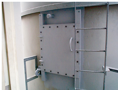
1. Access door was installed in the stack to allow installation and removal of the stack balloon in a few minutes
